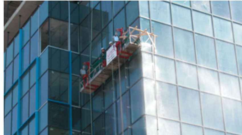
Figure 19: Calibrated sprinkler rack hung from suspended scaffolding
