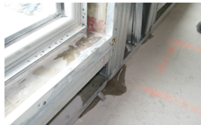
Figure 2: Example of water infiltration at a punch window assembly
