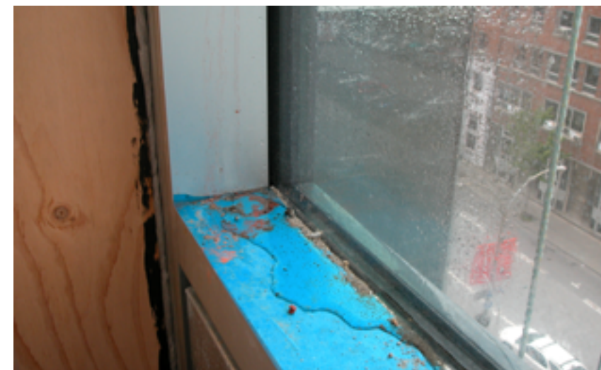
Figure 1: Example of water infiltration within a curtain wall assembly
